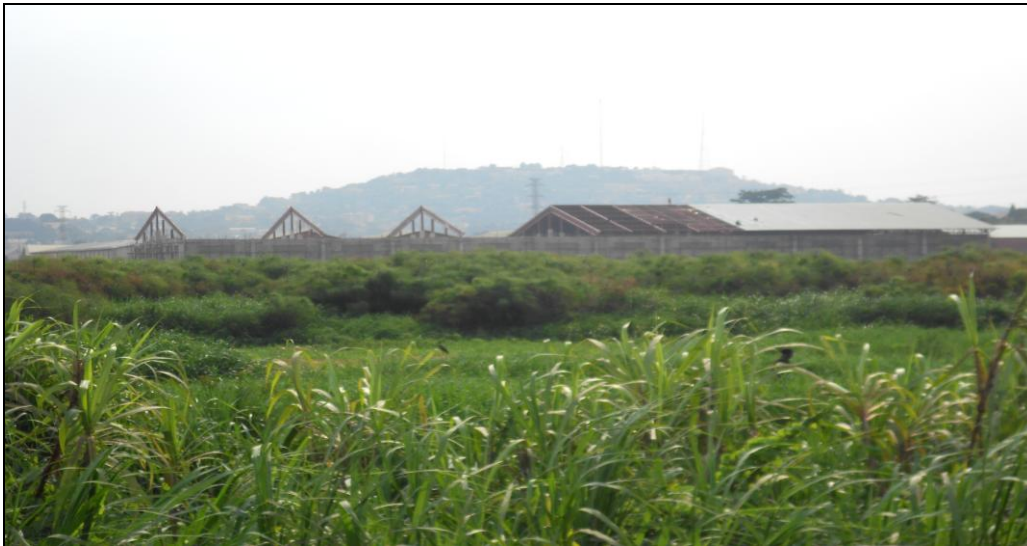
Fig. 5. An industry under construction in a reclaimed wetland near the Capital City – Kampala, in the Central Region, by Alex Barakagira, 2013
